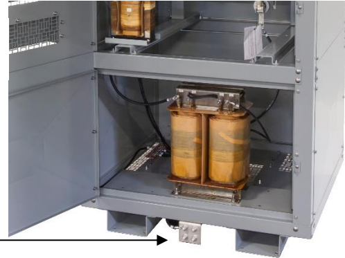
Ground Bus in a free-standing NEMA 1 enclosure
